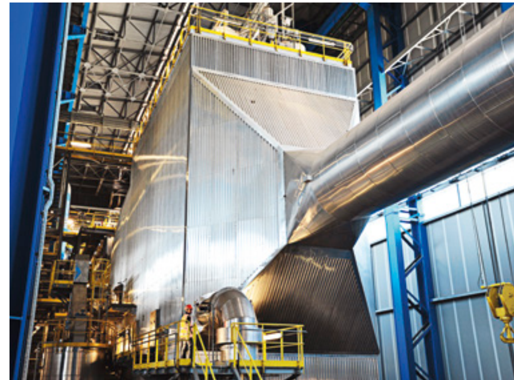
WASTE-TO-ENERGY PLANT IN TURIN, ITALY, BUILT BY CNIM.
