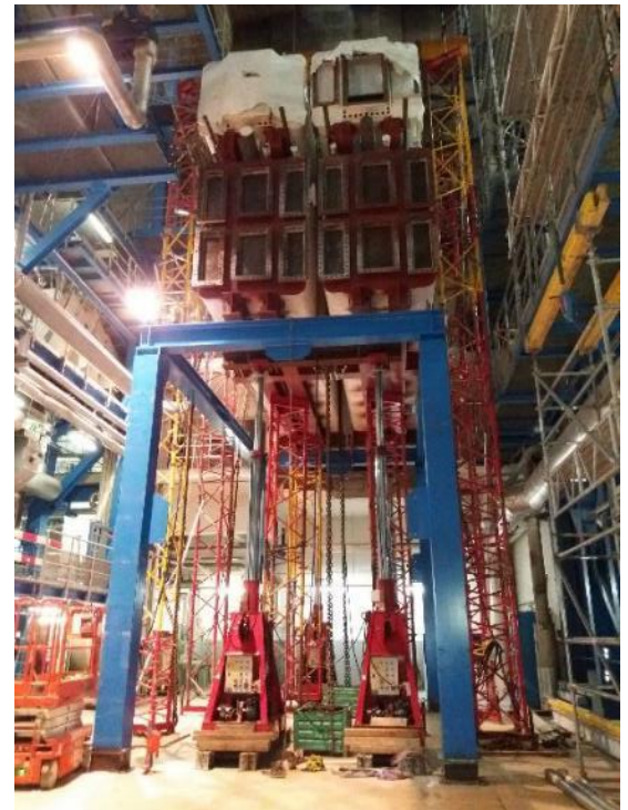
Basel Heat pumps
