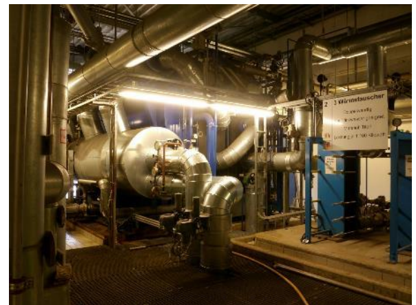
Erding Heat pump
